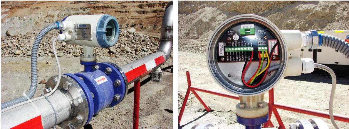
Capture flowmeter readings.
