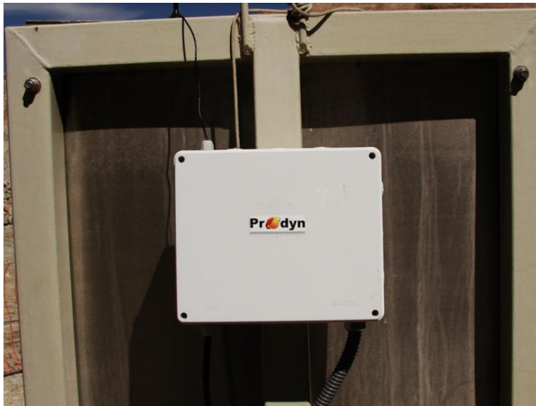
Box with data transmission devices
